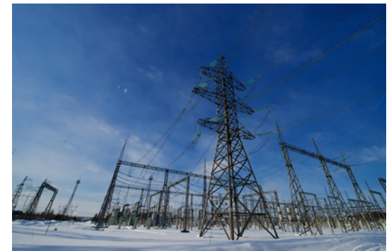
Substation 500 kV Tratchukovskaya
