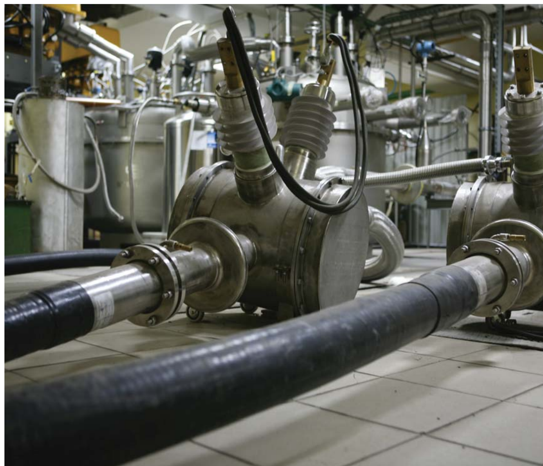
General view of the cryogenic station with current inputs of the cable line
