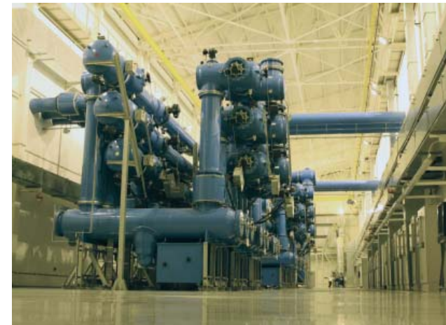
Fig. 3 Ochakovo 500kV substation is the Moscow Power Ring facility participating in the Energy Efficient Substation project
