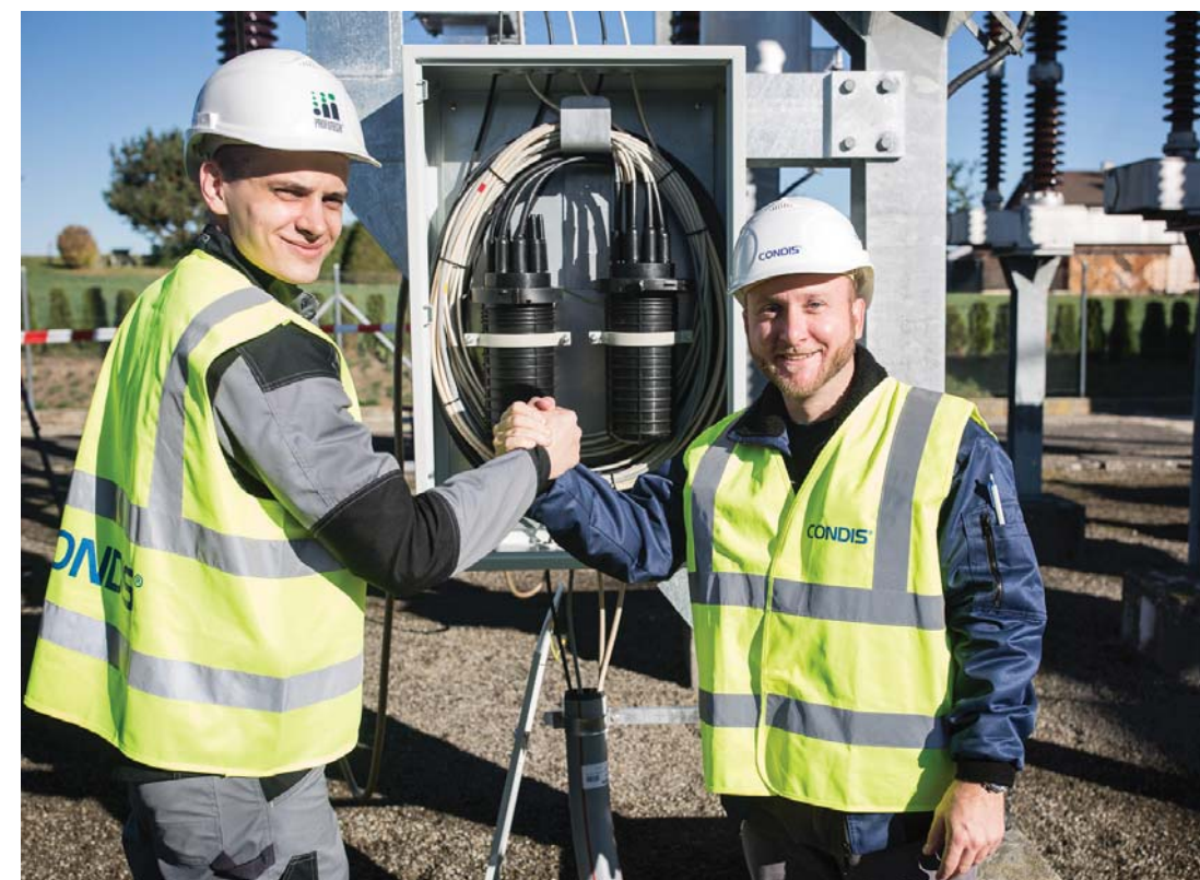
Fig. 2 Engineers Demid POPOV and Thomas Heid completed the installation of an electronic measuring transformer at the GROUP-E substation in Switzerland
