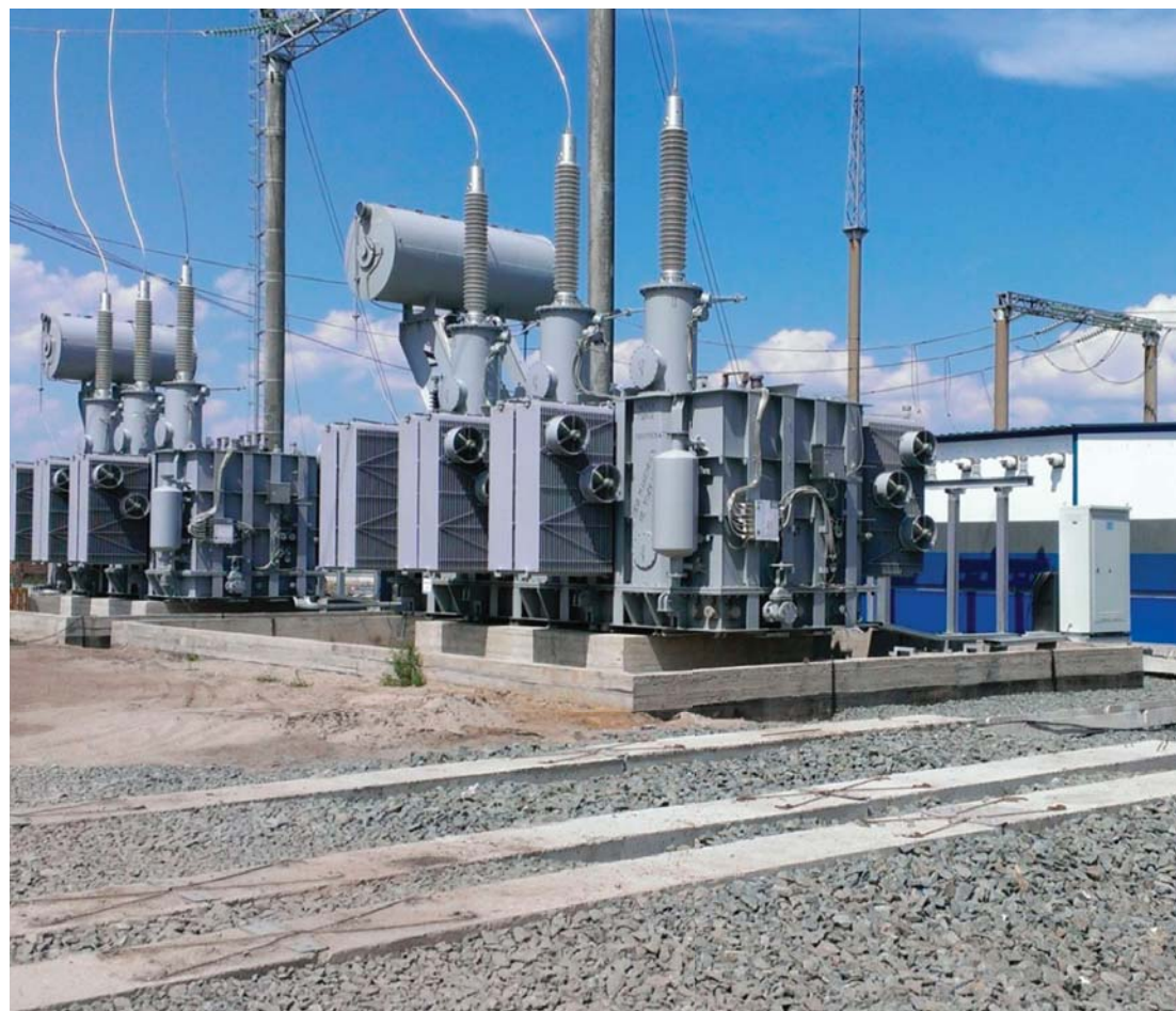
Exterior view of the TCR at the Svetlaya 220 kV substation
