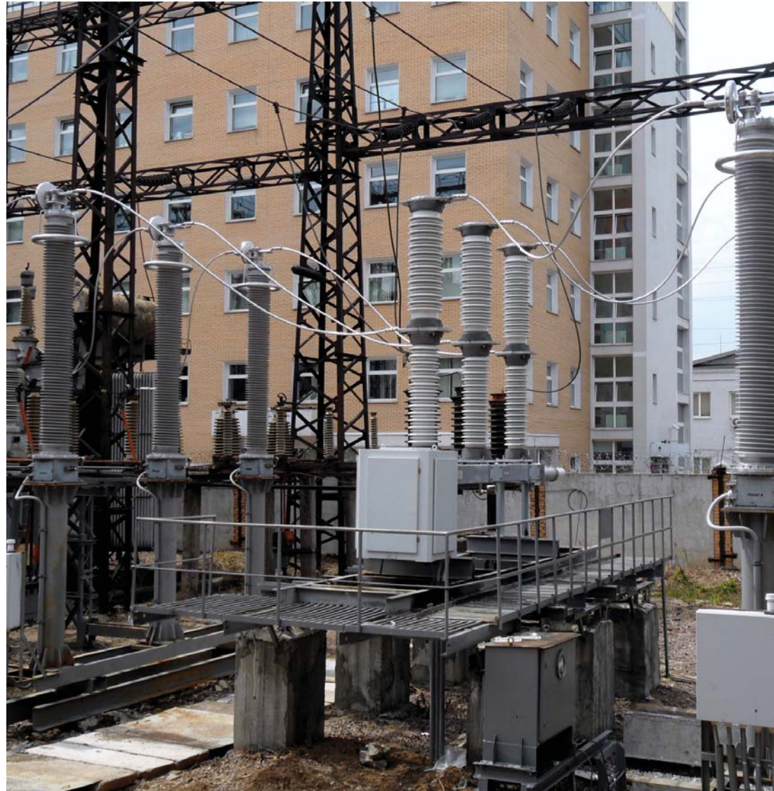
The optical transformers of the Digital Substation Test Site in R&D Center at FGC UES
