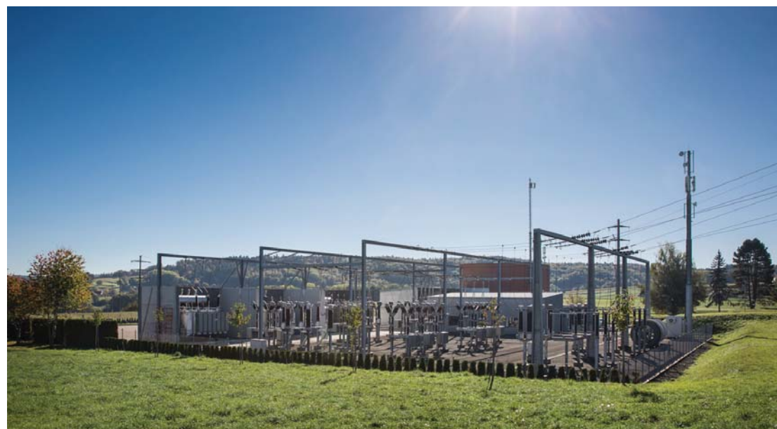
Fig. 1 The 3-phase combined NCIT is installed at the Villarepos Substation in Switzerland
