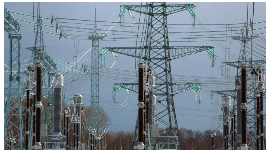
Fig. 1 Tobol 500kV substation is the first extra-high voltage facility in Russia where a package of digital technologies has been implemented
