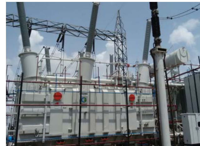
Fig. 3 The transformer with Izolyator bushings at PowerGrid 400 kV substation
