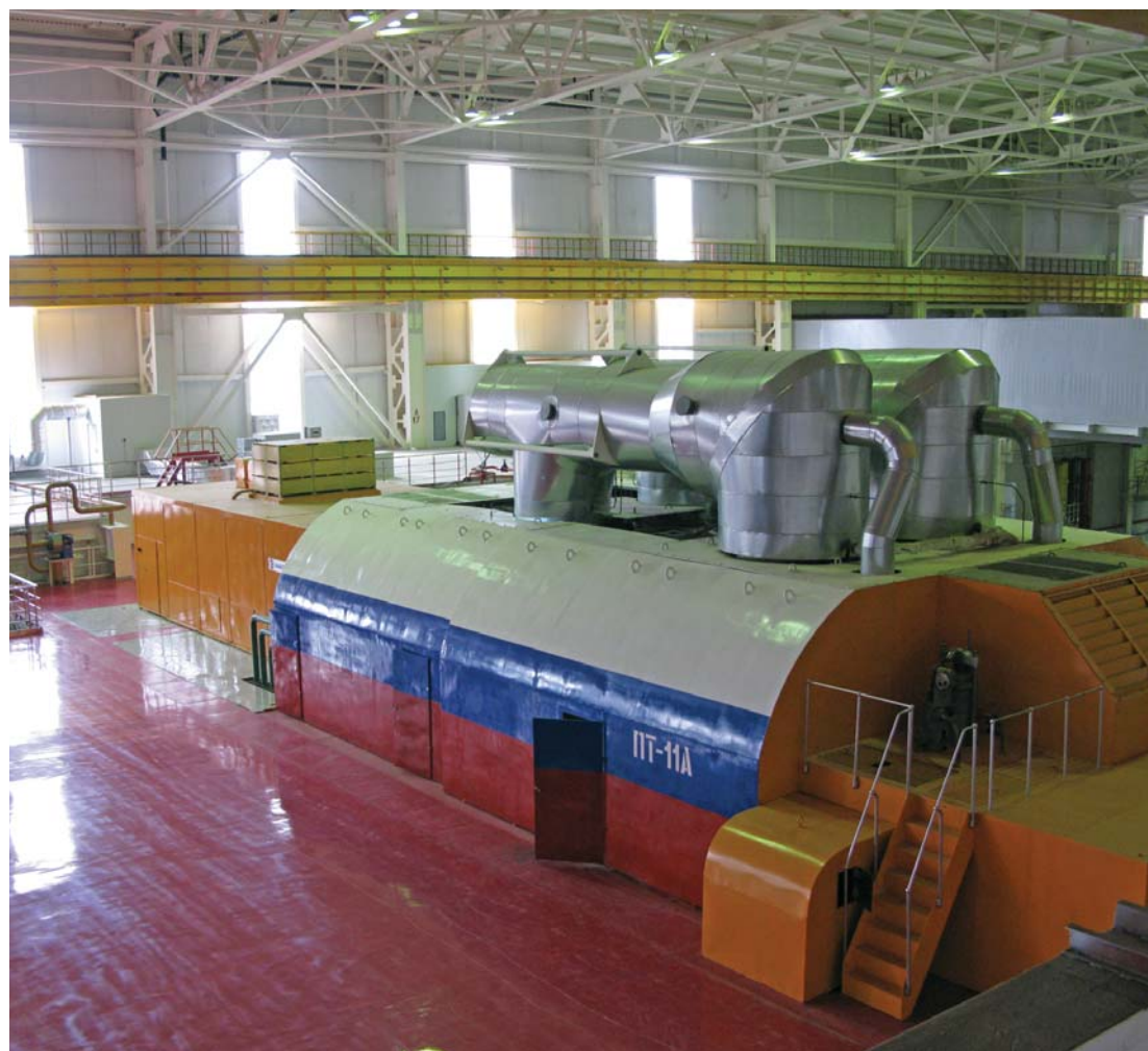
Asynchronized turbine generator T3FAU-160-2U3 with 160 MW capacity at unit 11 of CHP-21 by Mosenergo
